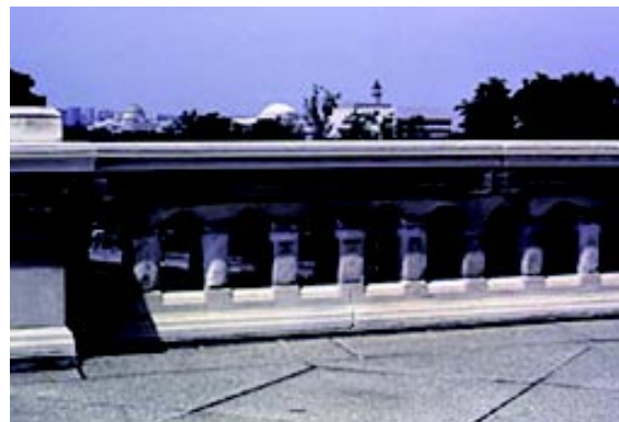
The marble balustrade on the west side of the Capitol building shows damage from acid rain dissolving the mineral calcite. 58
